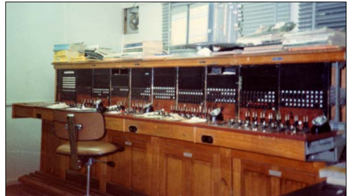
The Bowral Exchange switchboard in the 1960s
